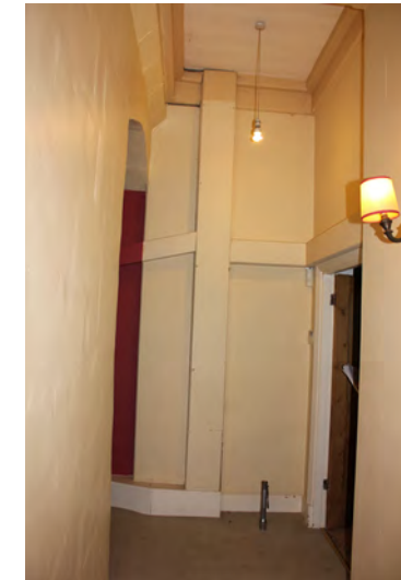
Modern boxed services in corridor
